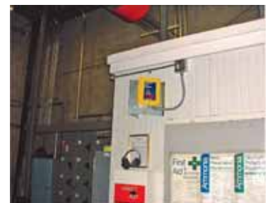
Ammonia leak detector installed in an engine room.
